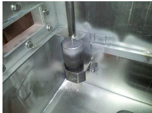
Wash tank float and tank overflow
