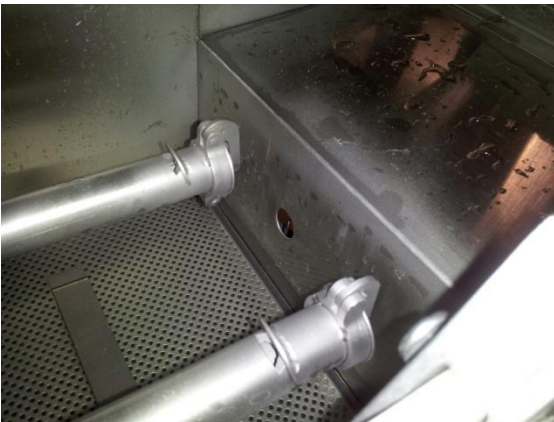
Showing hole at the side of tank, 7/8" detergent fitting
