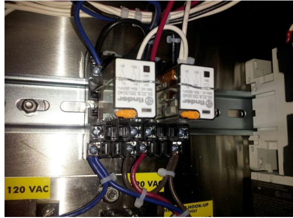
Conveyor motor control relays
