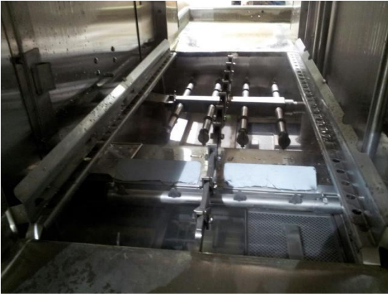
Travel through conveyor tray rails, center pull bar w/dogs
