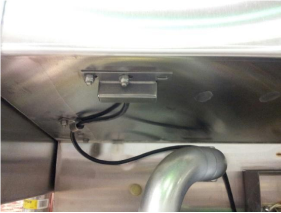
Sequence reed switch for wash tank
