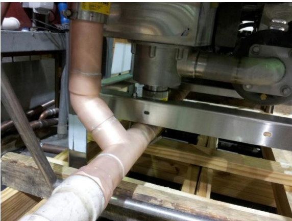
Showing 2" drain manifold exiting sump & scrap box
