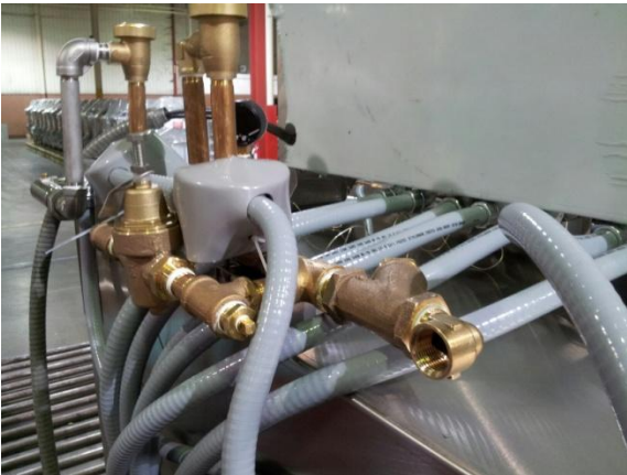
Hot water inlet manifold, single point ¾” pipe, PR valve
