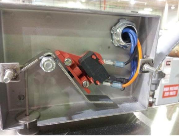
Showing “float” switch that controls fill water & heater
