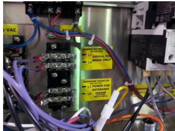
Dispenser signal connection terminals in control box
