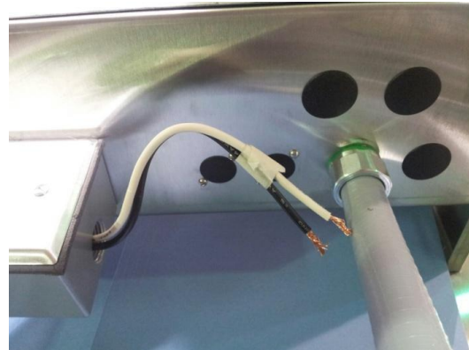
Showing power connection box for 120v wiring
