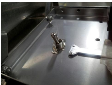
De-lime switch in control box
