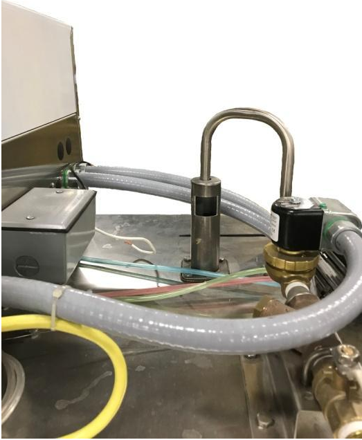
Showing 1/2" female pipe inlet, ball valve, y-line filter, water solenoid, ASSE approved air gap (backflow preventer)
