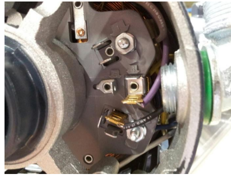
Line connection spades for L1, Neu (arrow 1 & 2)
