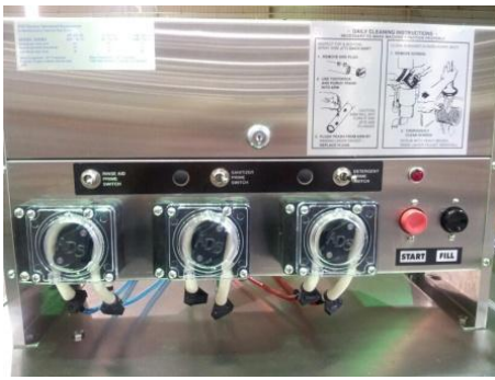
Showing deter, rinse, sanitizer external pumps
