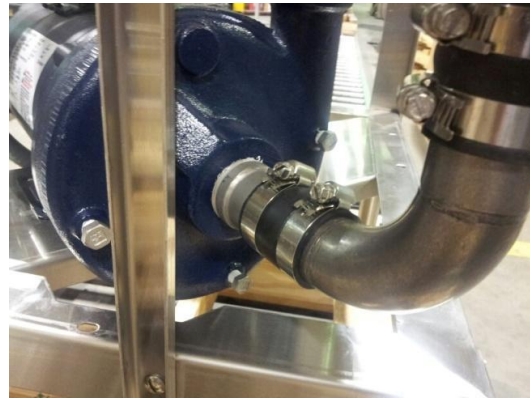
Pump intake and connector sleeves with clamps
