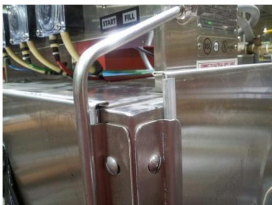
Showing misaligned arms
