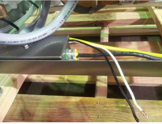
Power junction box for incoming 120v power
