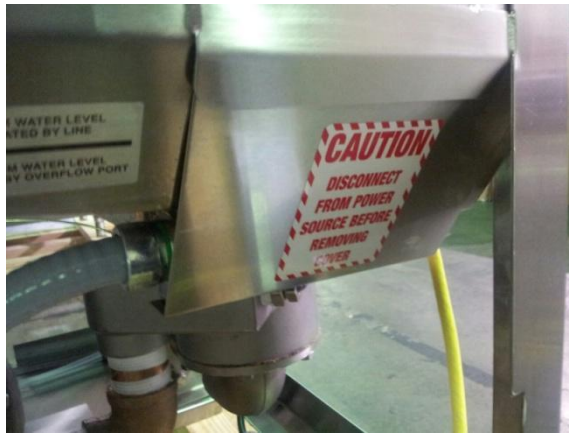
Heater terminal box in right front side of the pan
