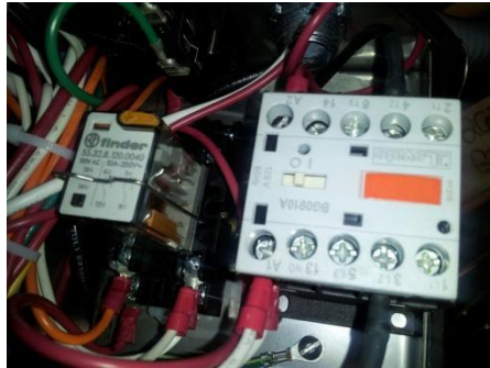
Left is Drain Relay, right is Heater Contactor
