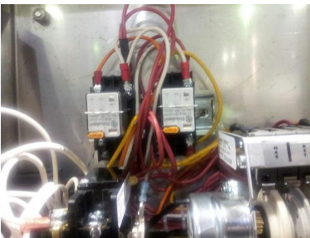
Left is Start Relay, right is Heater Relay
