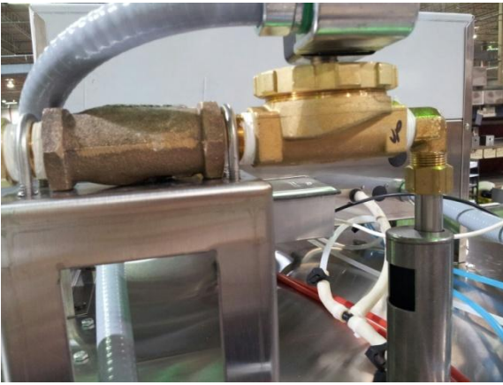
Showing the 3/4" pipe inlet, solenoid, and ASSE certified air gap.
