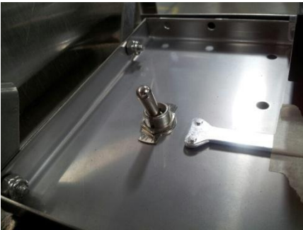
De-lime switch in control box
